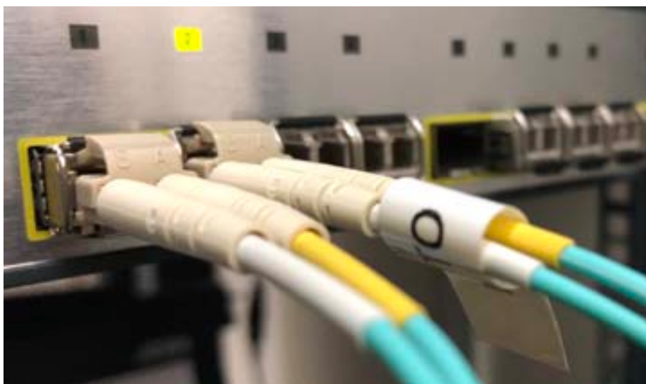
Fiber switch introduced for PAT systems communications.
